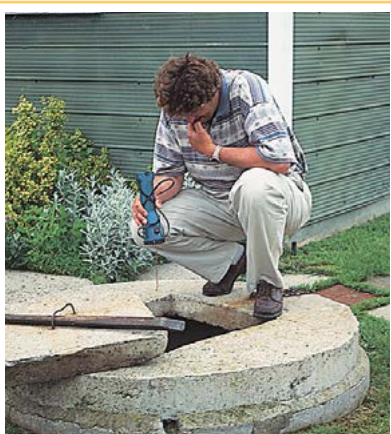
A visual inspection of the well cap should be part of your annual well maintenance program.
