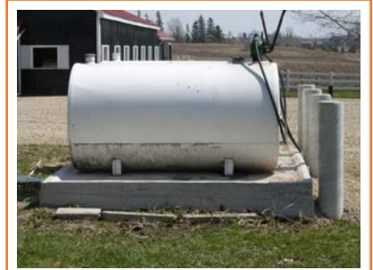
Locate fuel storage so it does not create a fire hazard for buildings.
