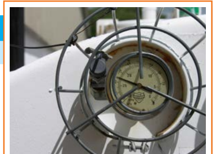
A vacuum reading indicates that both walls of a double-walled tank are sealed.
