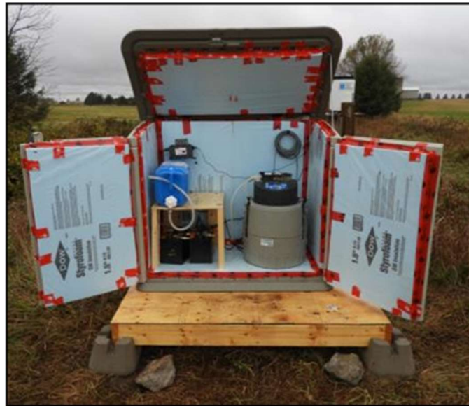
Figure 3. The inside of a water monitoring station established by the Upper Thames River Conservation Authority.
