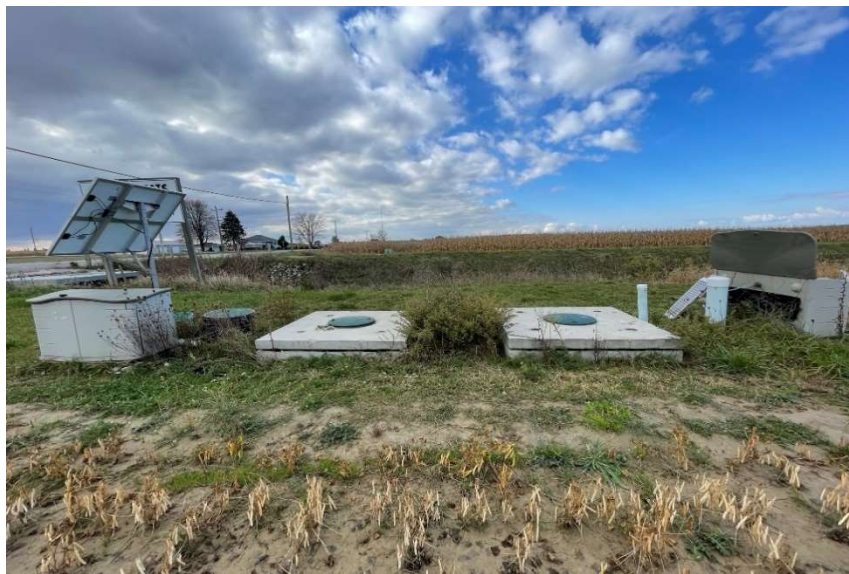
Figure 6. Fairview site containing an inflow permanent ISCO enclosure with solar panel [Right], first tank [Right Middle], second tank [Left Middle], and outflow permanent ISCO enclosure with solar panel [Left].
