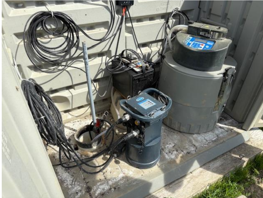
Figure 3. The inside of a water monitoring station established by Lower Thames Valley Conservation Authority (LTVCA).
